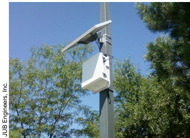
Figure 9. Photo. Example of a Bluetooth Antenna Installation.
