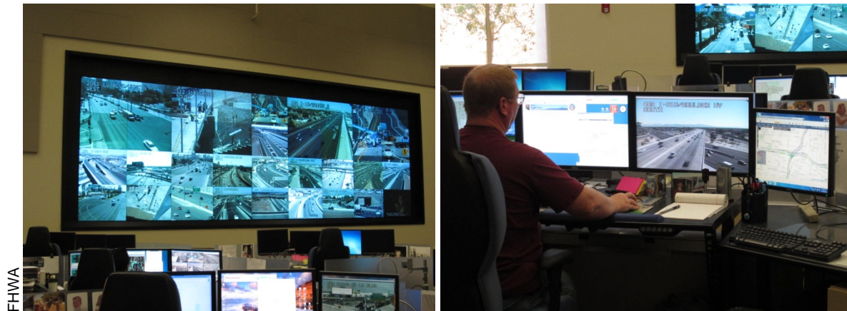
Figure 16. Photo. The Las Vegas FAST Control Room.
