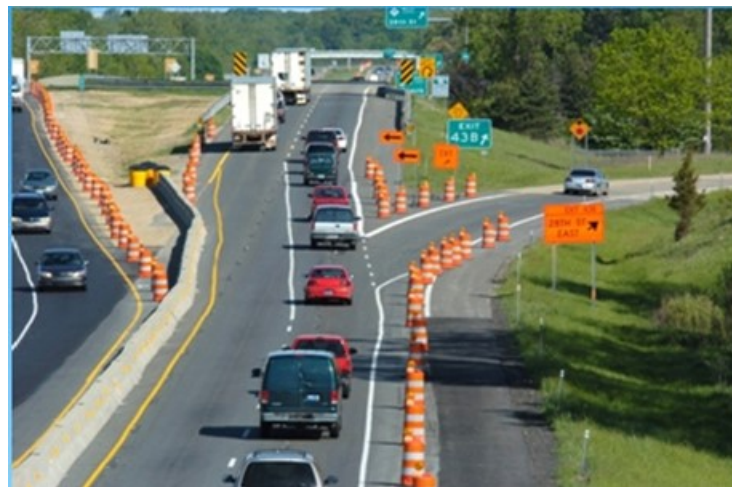
Figure 2. Photo. Example of work zone management activities. (Source: Michigan Department of Transportation)
