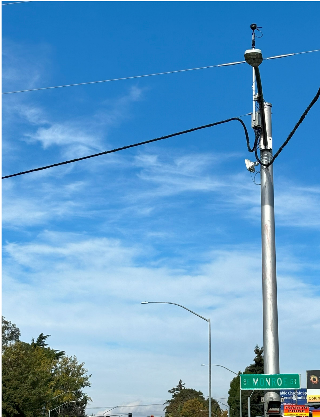
INSTALLED RADAR DETECTION
