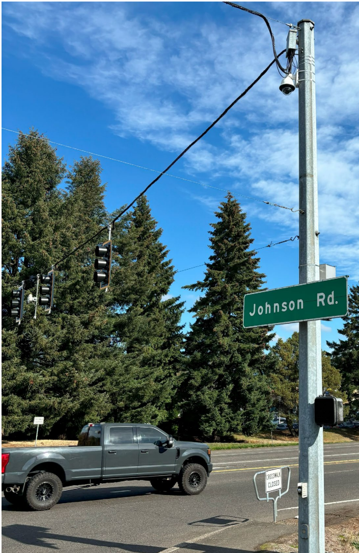
INSTALLED PTZ CAMERA
