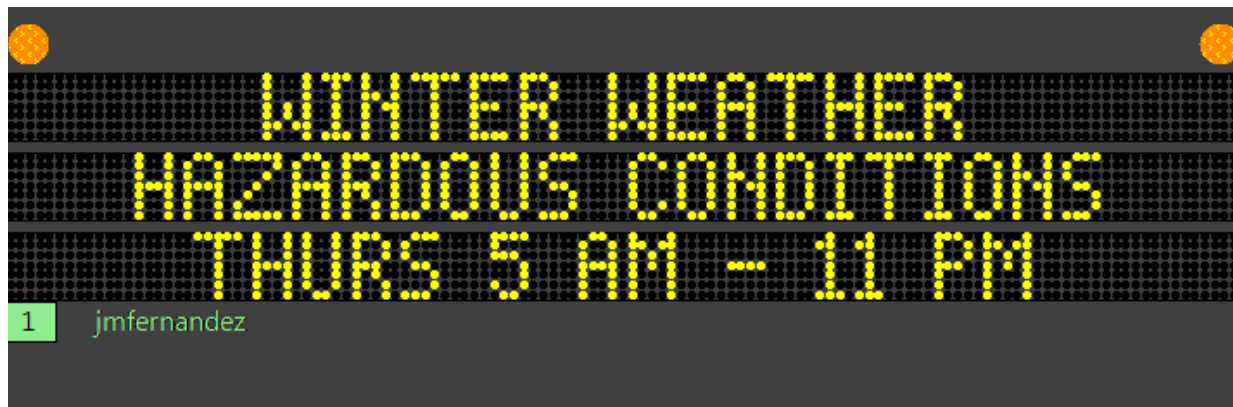
Figure 15. Photo. Wyoming Department of Transportation Traffic Management Center Dynamic Message Sign Updated 12/24/25. (Source: Wyoming Department of Transportation)
