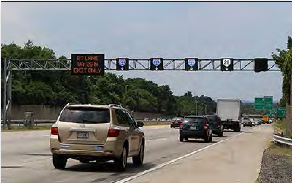
Figure 2. Photo. ATM installation on I-66, Virginia (Source: VDOT).
