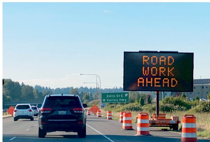
Figure 1. Photo. Portable changeable message sign in Washington State. Source: FHWA
