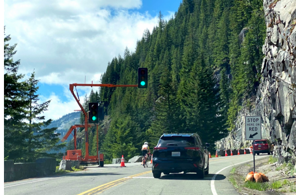
Figure 14. Photo. Temporary signal in Washington. Source: FHWA.
