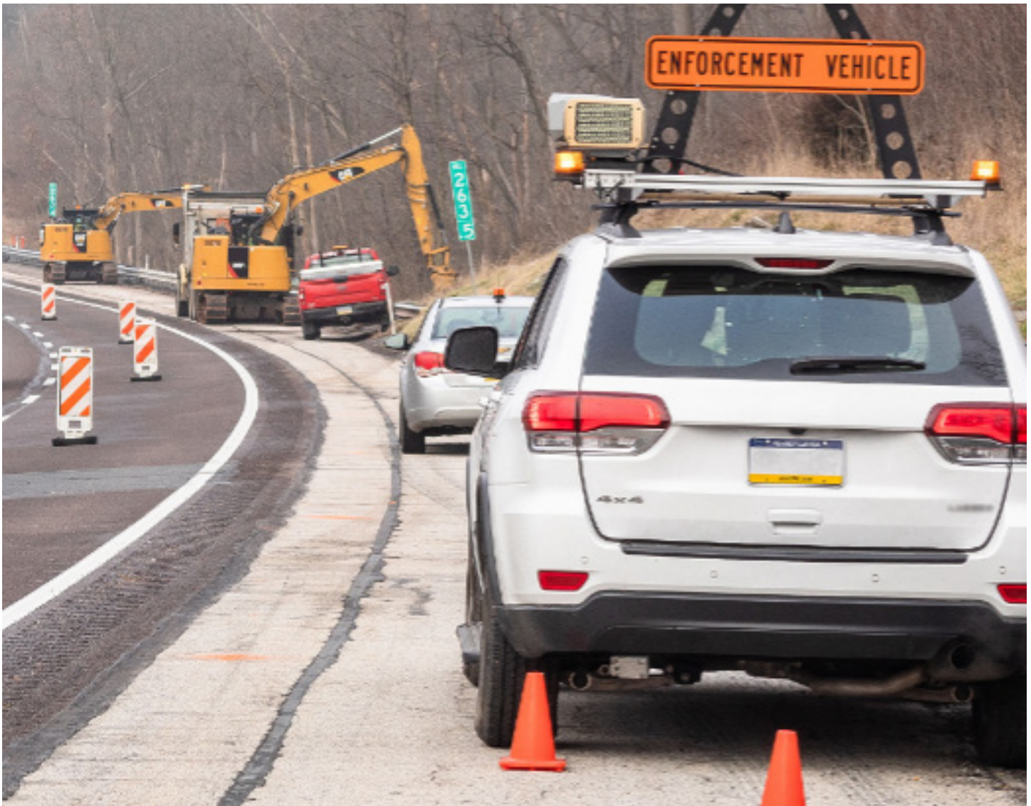
Figure 4. Photograph. Pennsylvania work zone speed safety camera enforcement vehicle in a channelized work zone. (Source: Pennsylvania Department of Transportation (PennDOT)).
